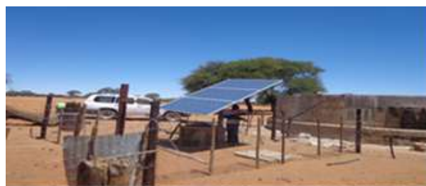
A Photovoltaic Pumping System produces energy for pumping water for livestock and domestic use.
