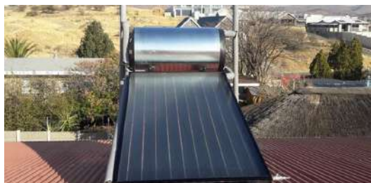
A Solar Water Heater uses energy from the sun to heat water for domestic use.
